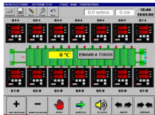
Temperature control screen
