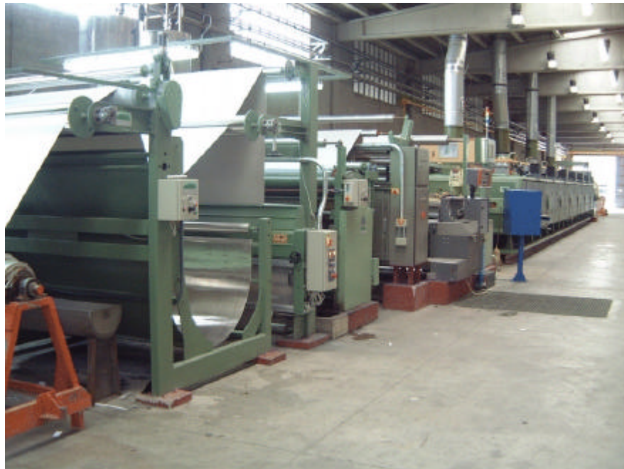
Drying and thermosetting unit 7 chambers
